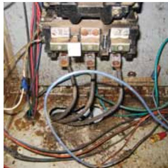
Corrosion leads to premature component failure
