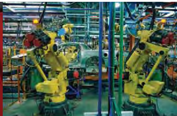
Process and Production Equipment
